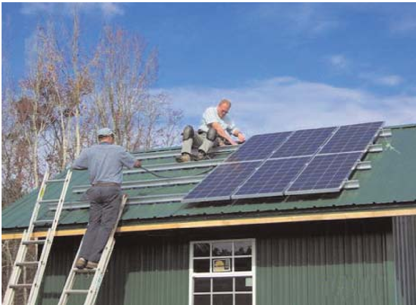
Solar panels on the roof of this shed will capture energy that will be used to operate an irrigation system.
